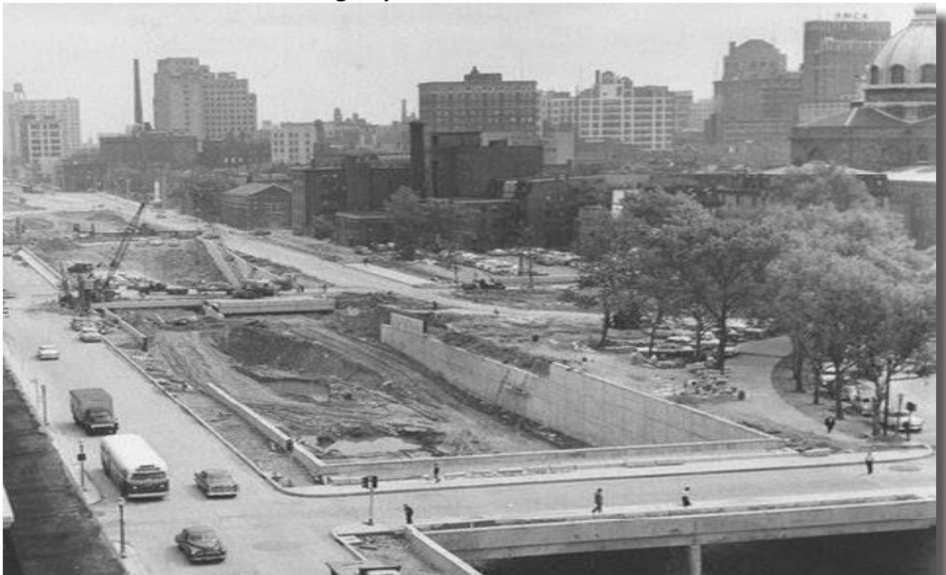
Figure 8 Intersection of Vine Street and 20th Street in September 1957 during construction, Source : PAHighways.com
