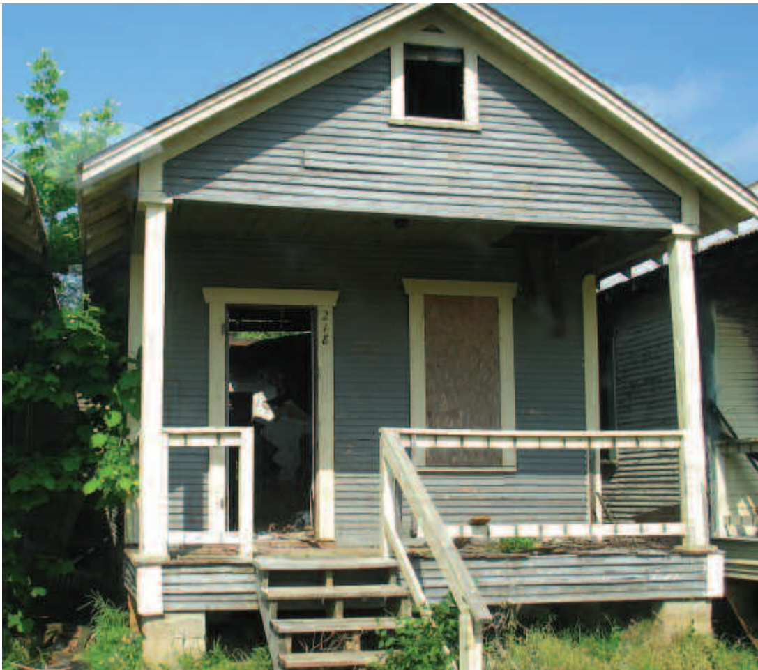
Shotgun-style homes dominate the Ledbetter Heights neighborhood. Re-creation of this indigenous housing style can help revitalize Shreveport.
