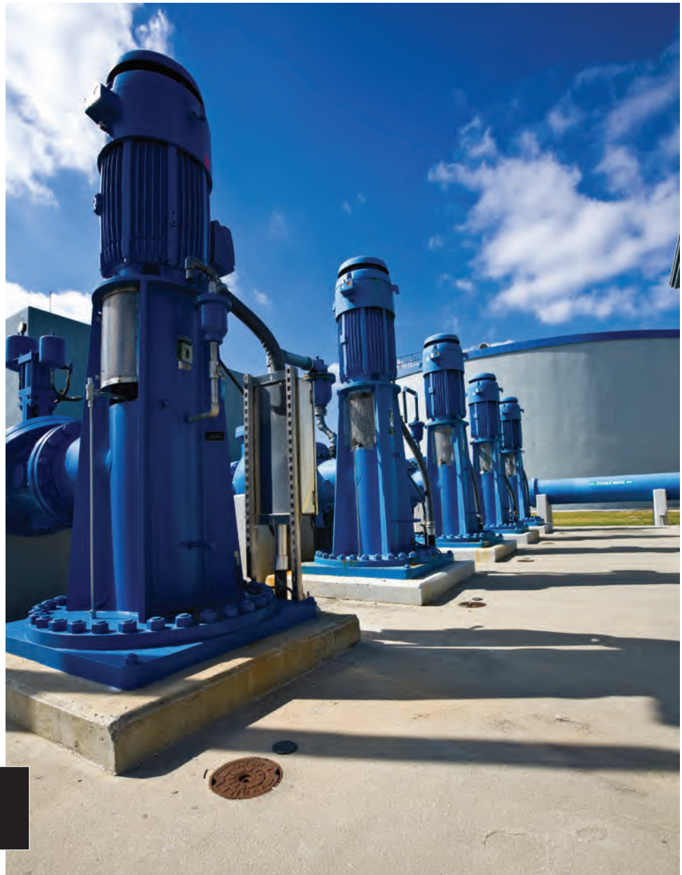
Water pumps at a purification plant are used to transfer freshwater from treatment units to storage tanks.
