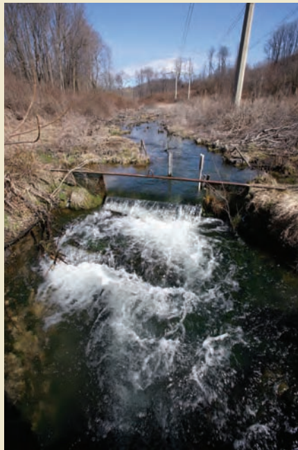
Marshland forms in Newburgh, New York, the result of a cracked underground concrete tunnel that is leaking millions of gallons per day. (AP)
