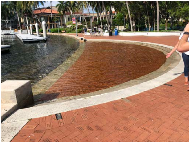
The site already has sunny-day flooding.
