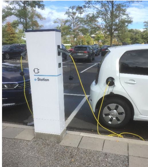
Electric charging point outside Autostadt.
