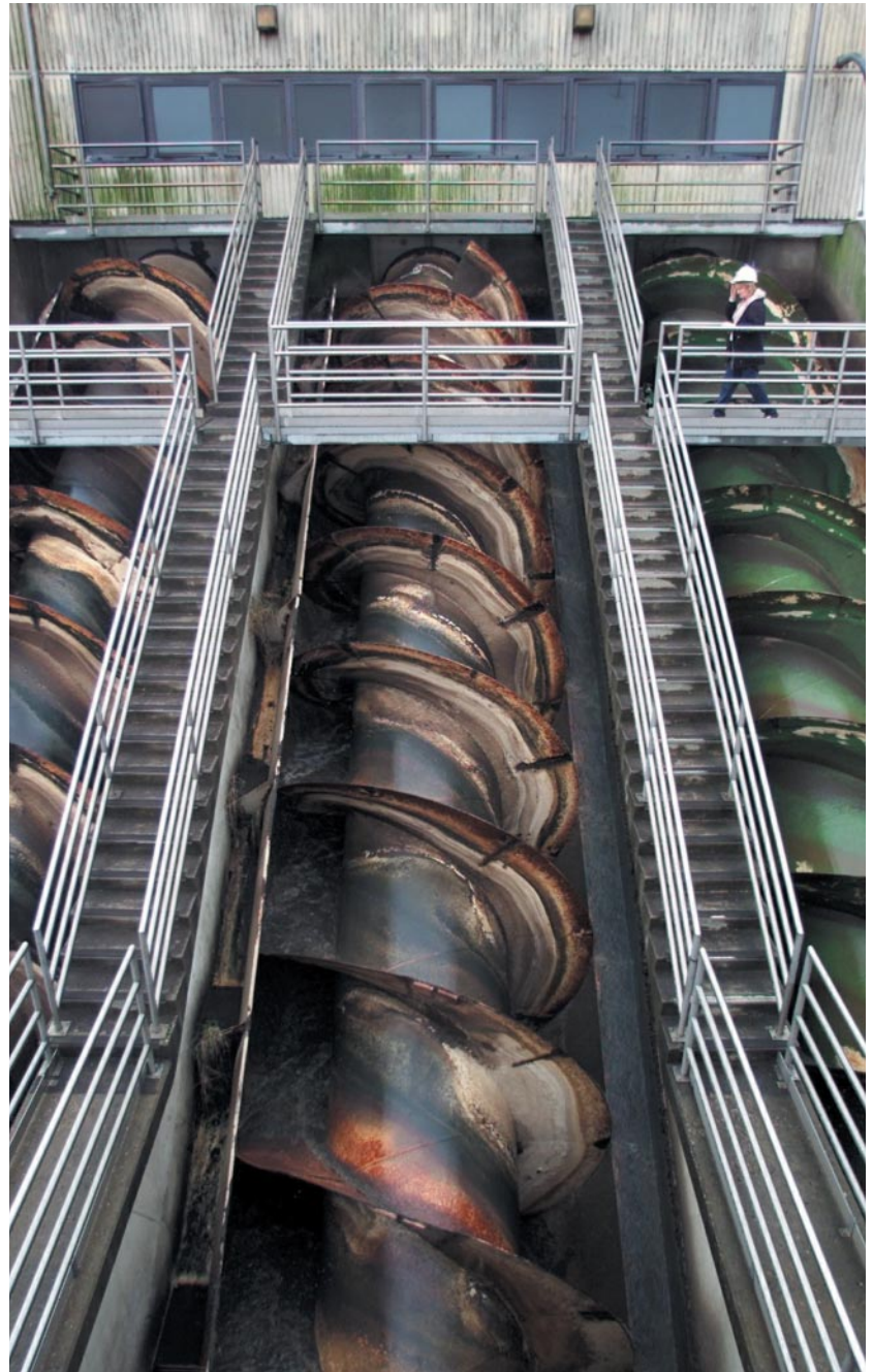
U.S. wastewater plants nationwide are in need of repair.
